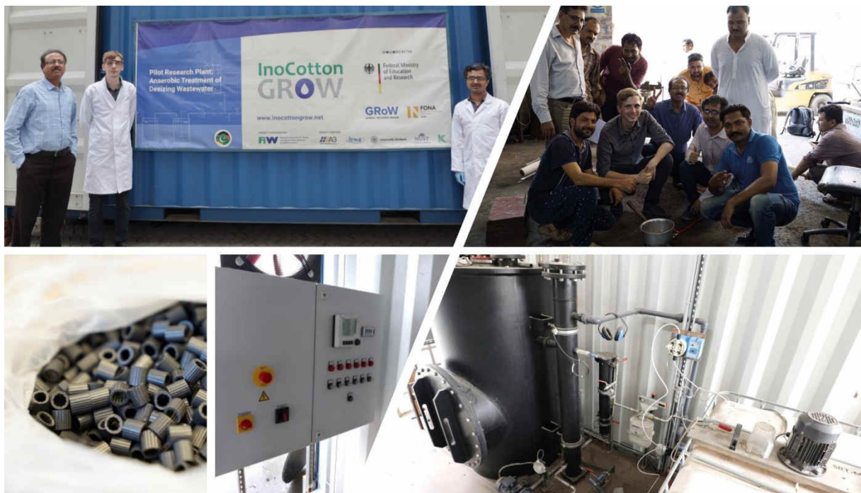
Figure 6.7: AnMBBR pilot-plant in operation at KML in Kasur producing biogas for water heating. © FiW
