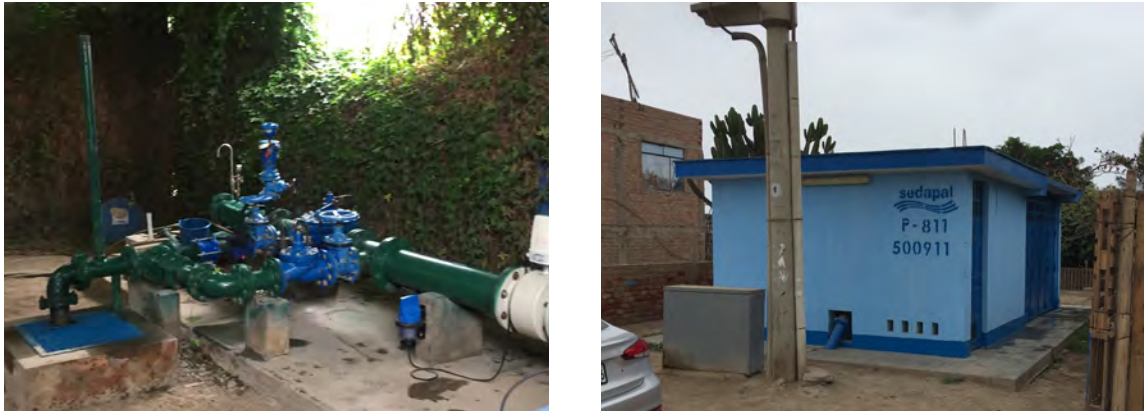
» Figure 5.4: Well head (left) and well building (right) of a SEDAPAL well. Pictures: S. Stauder.
